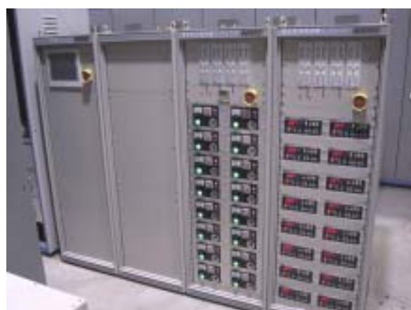
FIGURE 11. New controllers and power supplies for vacuum pumps and gauges
