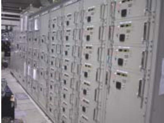
FIGURE 12. New magnet power supplies
