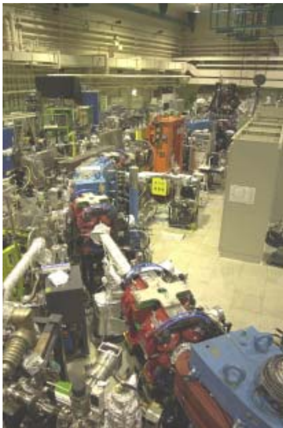
FIGURE 9. A part of the storage ring (between B02 and B04) just after finishing the installation. New in-vacuum undulator between B02 and B03, and a short free space reserved for future undulator can be seen.
